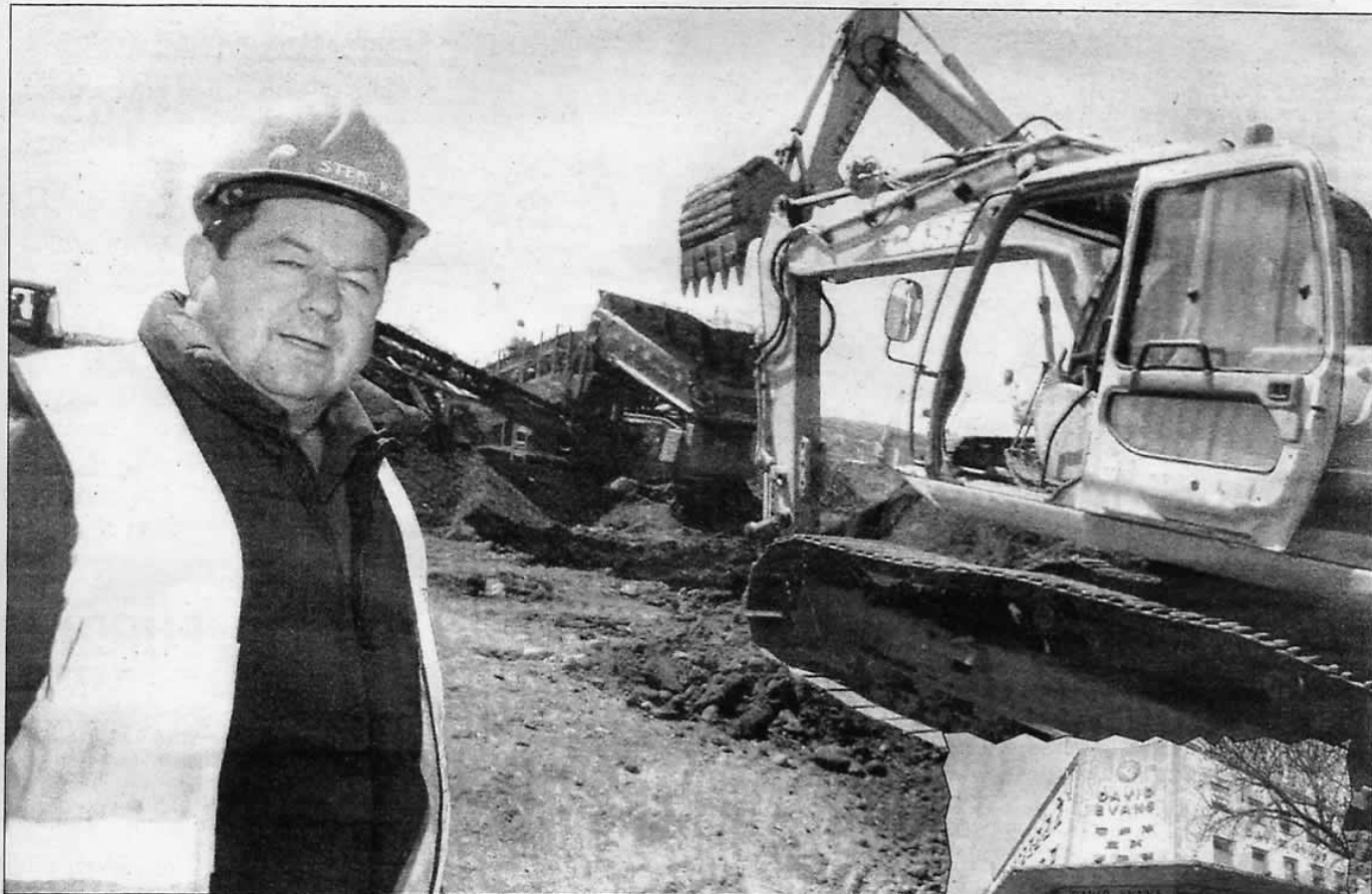
STONE ME Steve Norman of Stenor (above) on site where the rubble from David Evans is being processed, and the store in its former glory (right).
